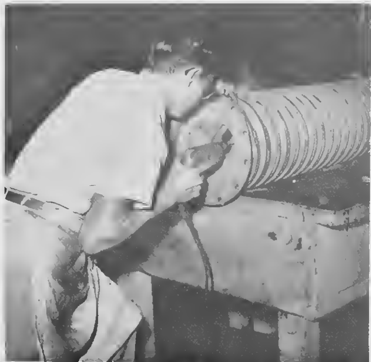
WITH A pistol-grip electric drill, B. Tromp, tradesman B, drills holes for set screws in an expansion joint. CU UN drill electrico di man, B. Tromp, tradesman B, ta drill buraco pa schroef den un expansion joint.
